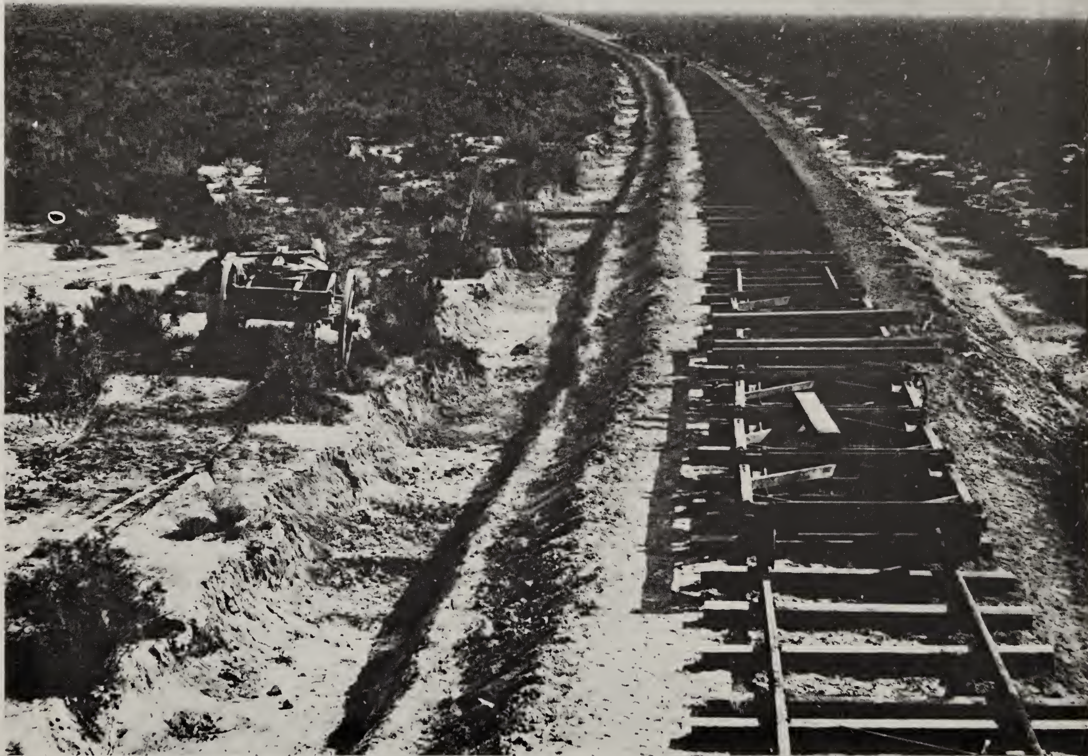
Figure 11: Track laying in the Utah desert (Southern Pacific, Alfred A. Hart Photograph).
